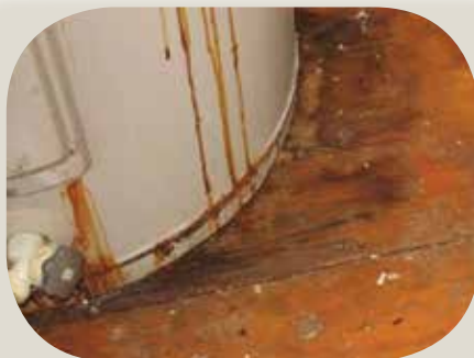
Leaky water heater
