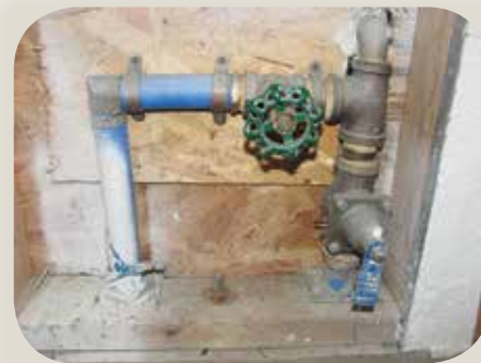
Main shutoff valve
